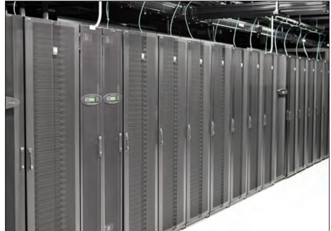
A combination of custom GF-Series GlobalFrame Cabinets provided the backbone for implementing a complete CPI Hot Aisle Containment System (HAC) solution for Cologix, Inc.
